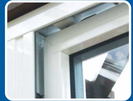
Secure Night Vent Facility
